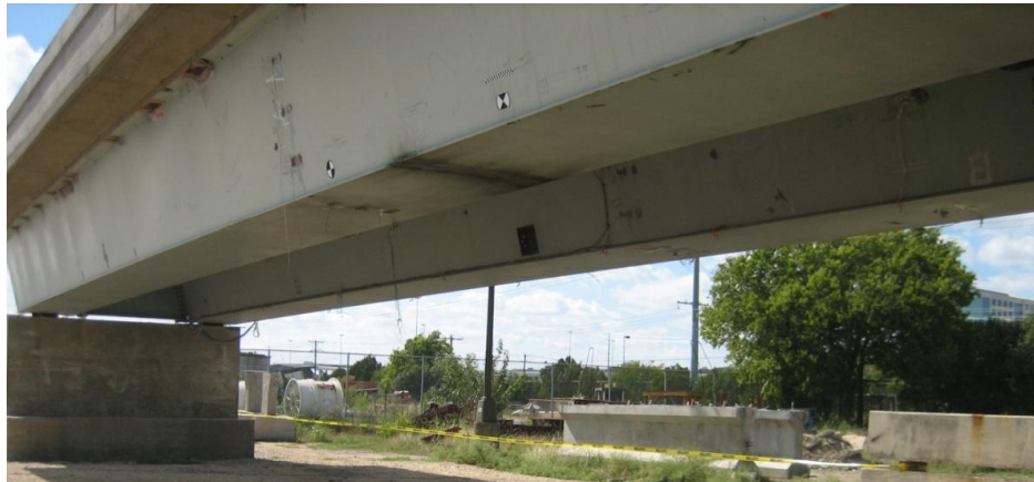
Figure 4. Bridge fracture after explosion.
