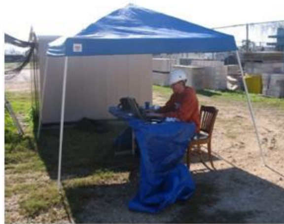
Figure 13. Remote load cell monitoring.
