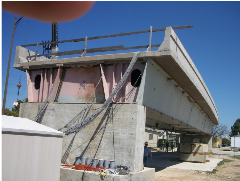
Figure 5. Wires connected to instrumentation
